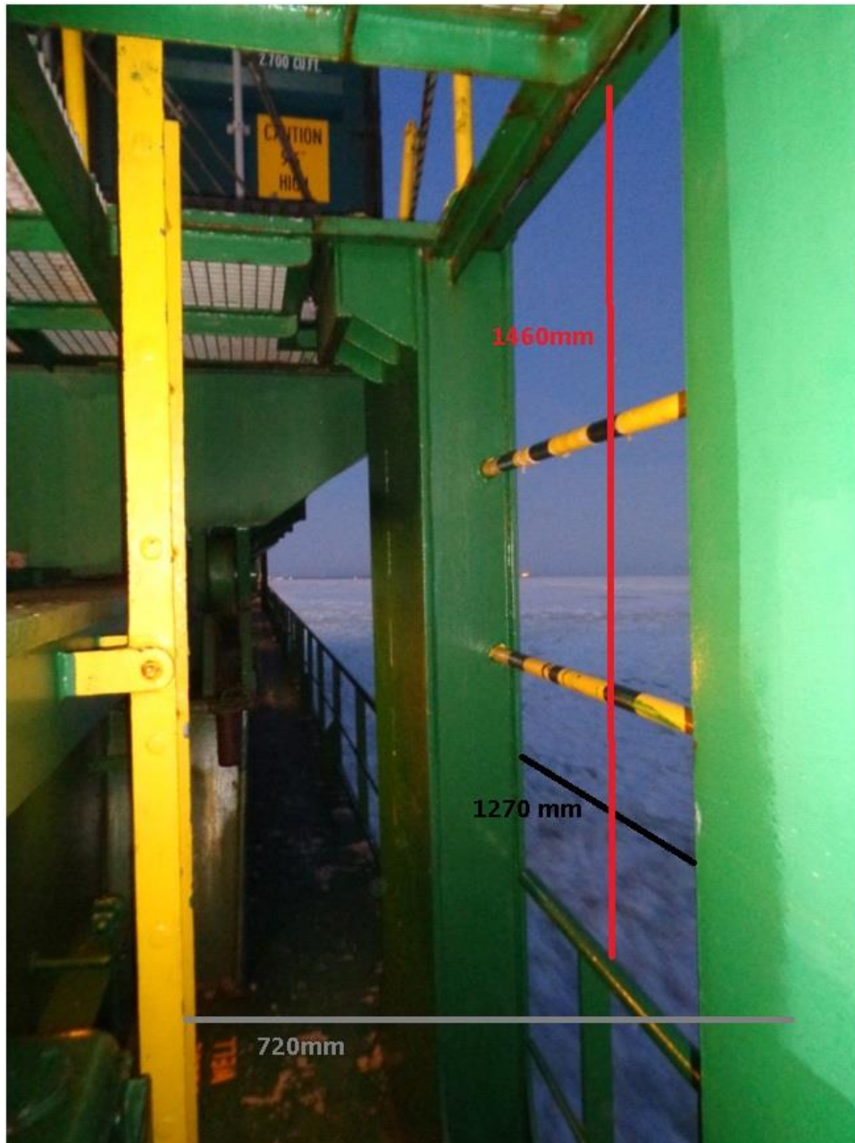
Figure 12. The picture shows the distance between the ladder and the railing (720 mm) and the measures above the railing (1460 x 1270 mm) before the protection was mounted. The black-and-yellow pipes on the right hand side of the picture is the new protection, mounted after the occurrence. Image: Nordic Hamburg Shipmanagement (HK) Ltd.
