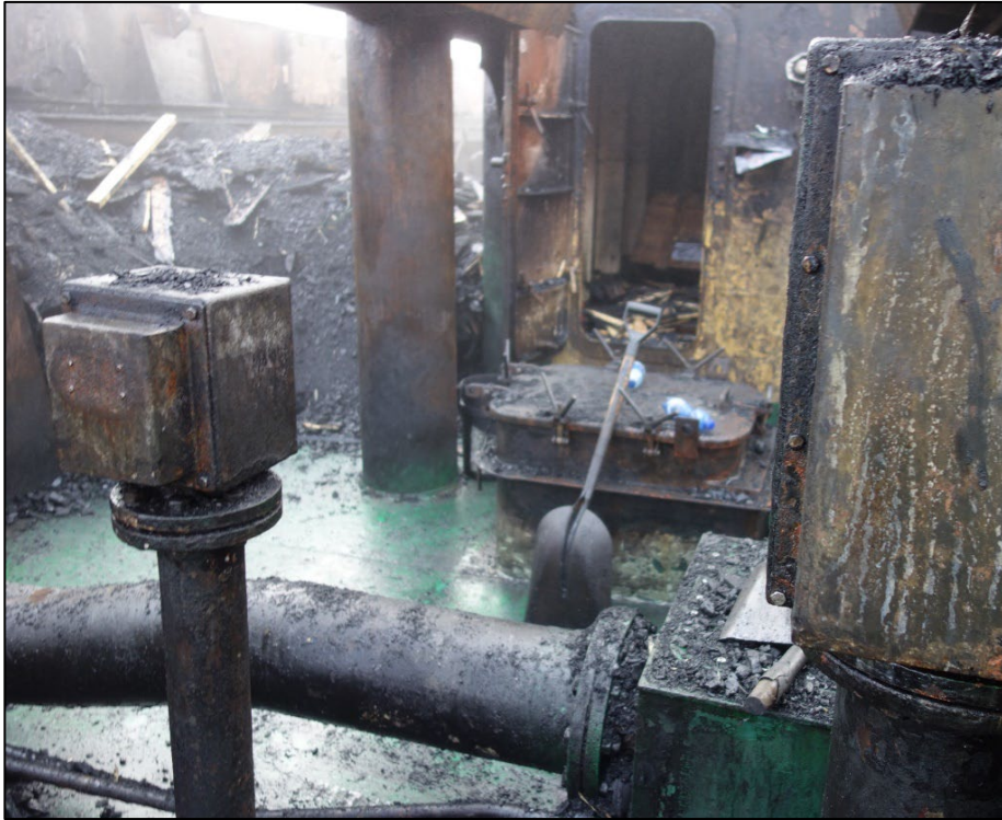
Figure 18. The port side deckhouse by crane 1 and the deck surface under the support structure for the cargo after the area had been cleared of carbon residue. The open door to the deckhouse is in the background.
