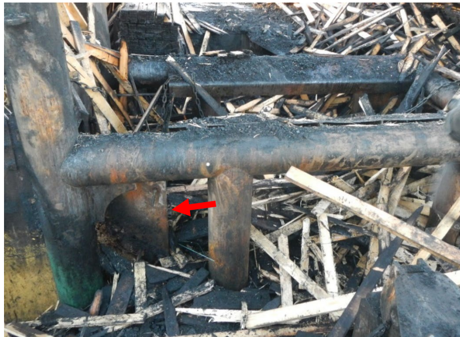
Figure 17. The support structure for the cargo by the port side deckhouse. The arrow marks the open door to the deckhouse.
