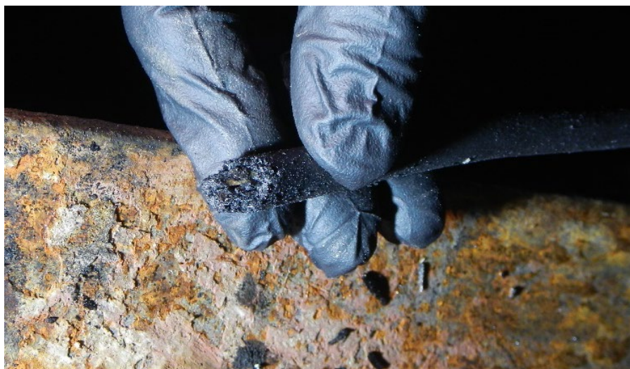
Figure 71. The torn off end of the extension cable that was plugged into an electrical outlet in the deckhouse on the port side of crane 1.
