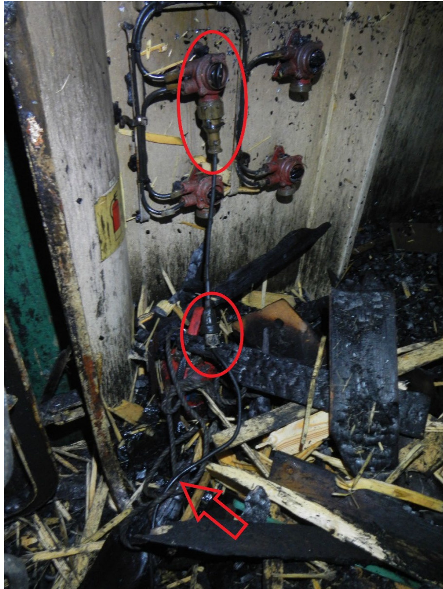
Figure 19. Shown in the upper ring is the electrical outlet with the switch in the 'on' position and the plugged-in extension cable in the deckhouse. In the lower ring, a connection can be seen between the cable from the electrical outlet and the extension cable that was out on the deck. The arrow points to the extension cable where it runs through the open door to the deckhouse on the left of the picture.
