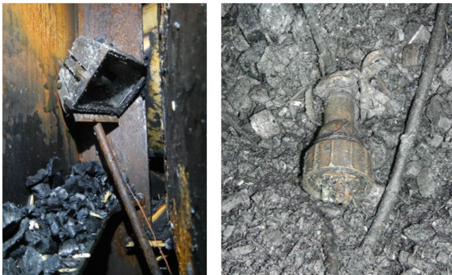
Figure 23. Portable floodlight that was leaning against one of the stanchions of the support structure on the port side of crane 1. The picture on the right shows the plug for the floodlight, which showed no signs of being plugged into an outlet during the fire.
