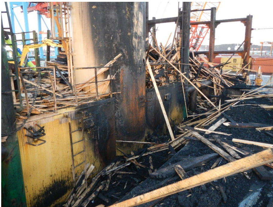
Figure 16. The deckhouses beside crane 1, with the port side deckhouse to the right of the base of the crane. The areas where the paint was burned off were larger forward and on the port side of the crane.
