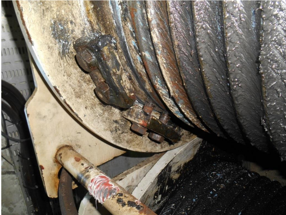
Figure 11. Cable locks on the winch drums. Image: Bulkship Management
