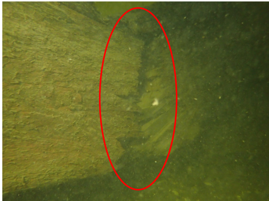
Figure 10. One of the three broken crossbars in the supporting structure. Image: Stockholm Vatten.
