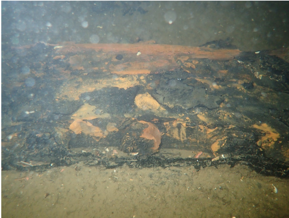
Figure 11. The water pipe's bolted flange at a joint and surrounding crush damage in the pipe. Image: Stockholm Vatten.
