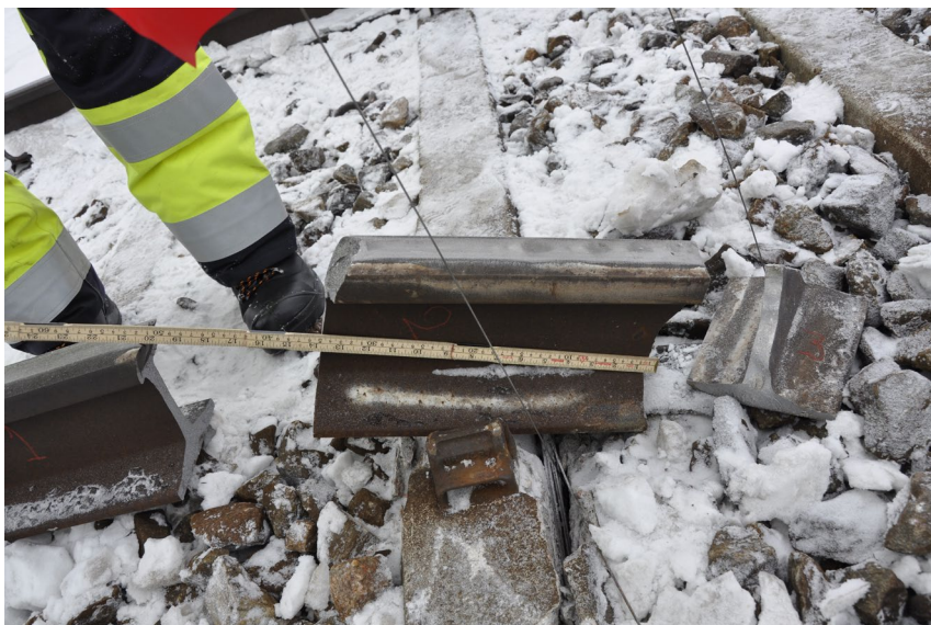
Figure 7. White spray paint on one of the pieces of broken rail.
