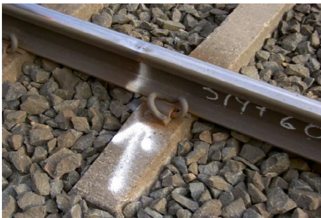
Figure 32. Excerpt from Infranord Mätenheten's work instruction Manuell OFP av räler och rälskomponenter i spår . Example picture of how to mark a defect that do not spread out along the length of the track. Source: Infranord Mätenheten
