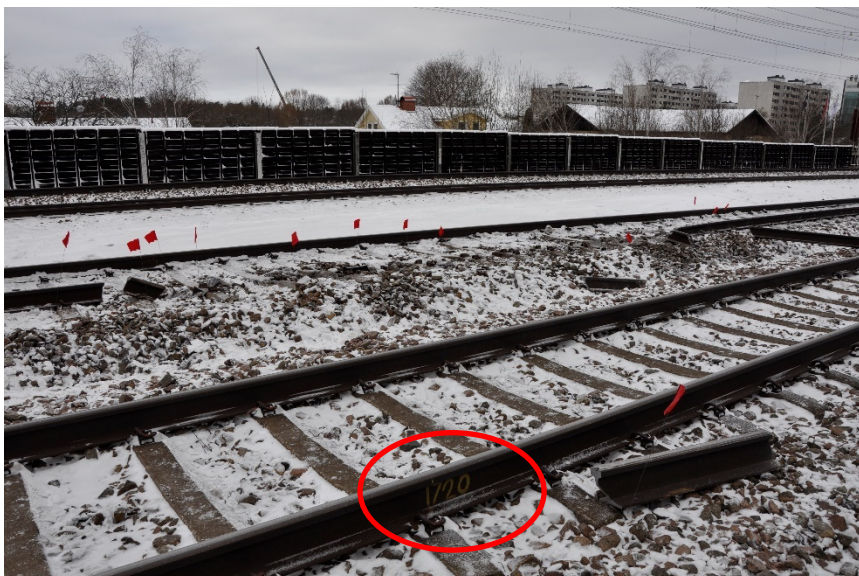
Figure 8. Adjacent rail marked with 720 in yellow paint. Corresponding marking was also found on one of the broken pieces of rail (see Figure 16).
