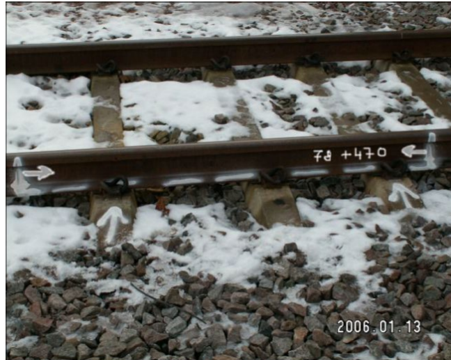
Figure 33. Excerpt from Infranord Mätenheten's work instruction Manuell OFP av räler och rälskomponenter i spår about how defects that are spread out a lot are to be marked on the installation. Source: Infranord Mätenheten
