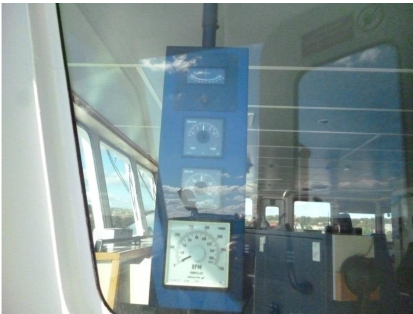
Fig. 2, Panel with indicators that can be turned to face the bridge wing.
