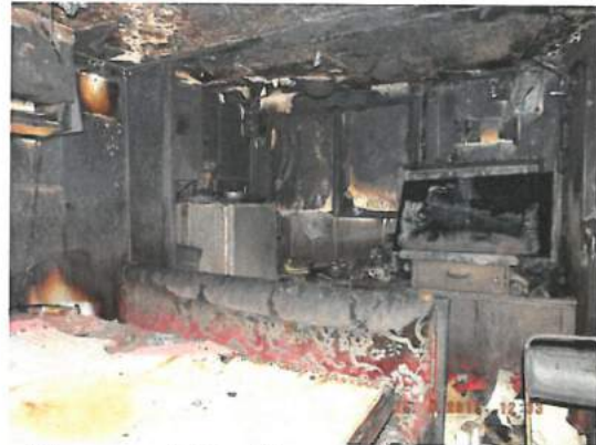
Photograph 23: Thermal destruction in the mess room
