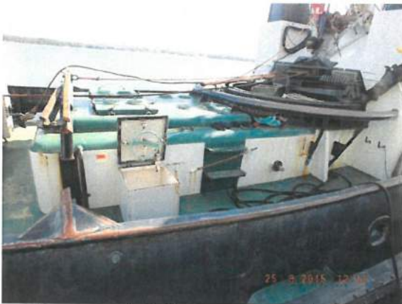
Photograph 6: Emergency exit from the engine room at the stern of the tug boat
