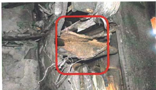
Photograph 14: A hole after burning of the bunk lamp over the top bunk bed in the watch officer's cabin
