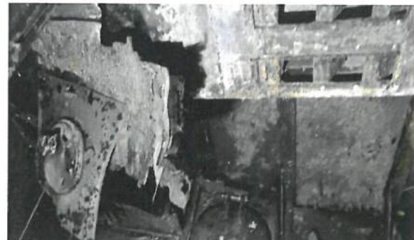
Photograph 17: Completely burned out ceiling in the central cabin on starboard side
