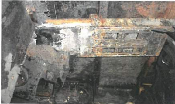
Photograph 16: Burned soot around the air inlet in the ceiling ventilation duct
