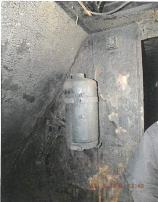
Photograph 30: Fire extinguisher at the stairs
