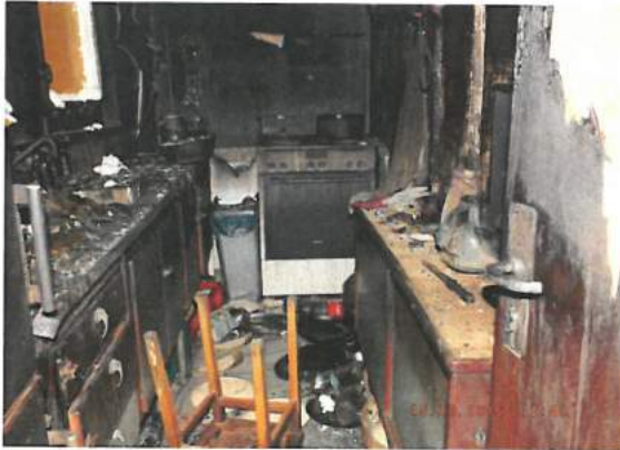
Photograph 22: Thermal destruction in the galley
