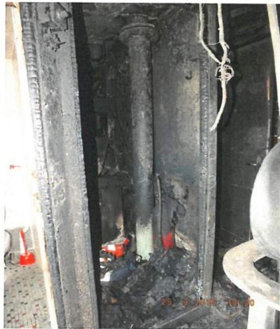
Photograph 25: Destroyed fire locker
