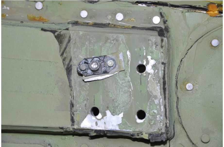
Photo 7: Internal view of the fairing showing the remaining screw, fastener and attached failed piece of bracket.
