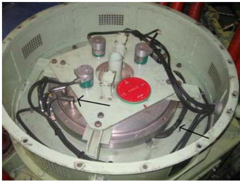
As original. Arrow on the right showing the control cables coming from underneath the pod and connected to the gauss. Arrow on the left showing the control cable connected to the otherside of the gauss and continuing to control units.
