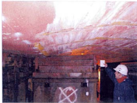
10. View of bottom damage
