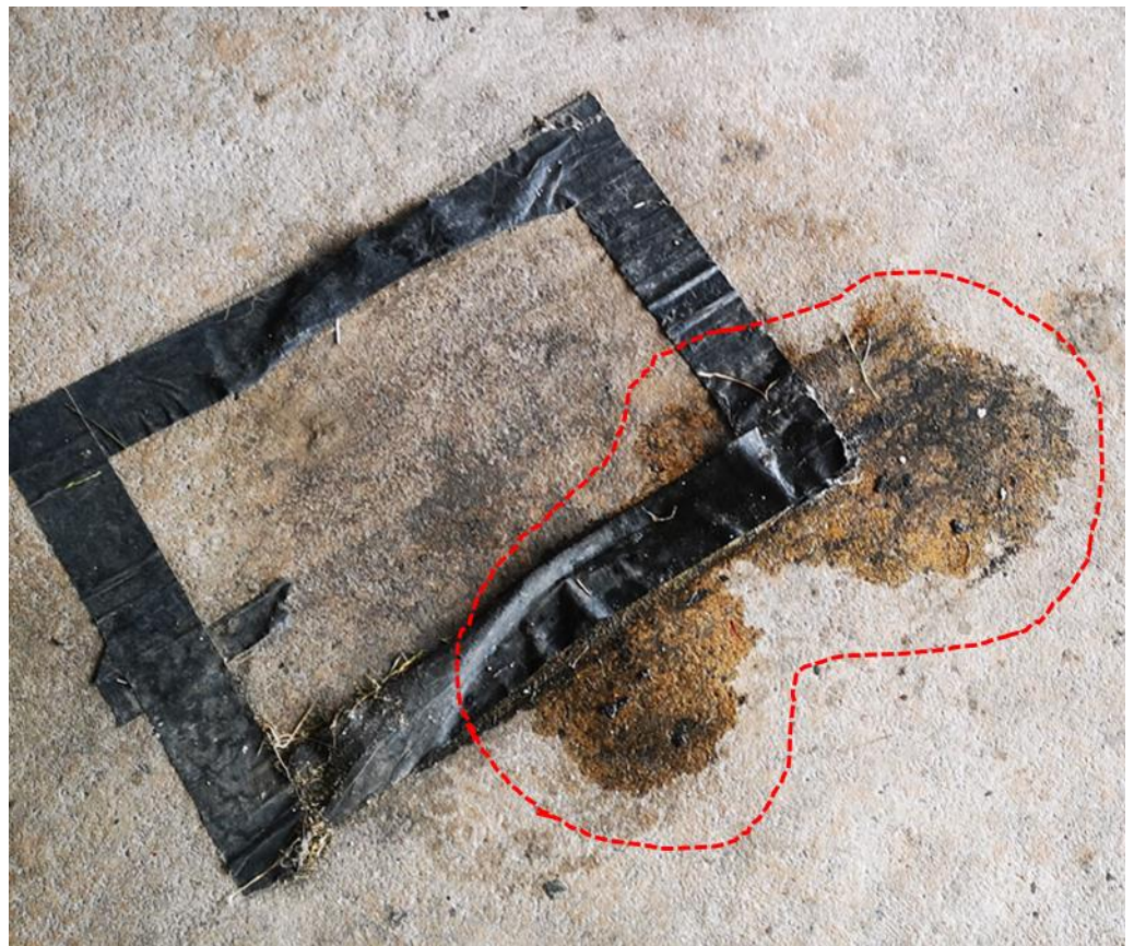
Figure 16. Stain on the hangar floor. Picture: The Pilot.
