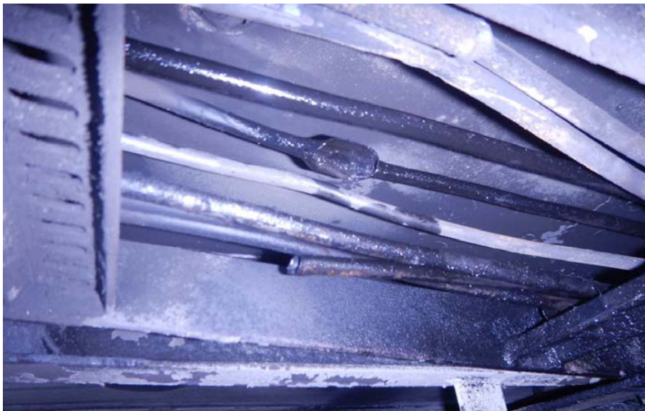
Figure 28. Lines for hydraulic oil and cable ducts above the cars, which were affected by the fire.
