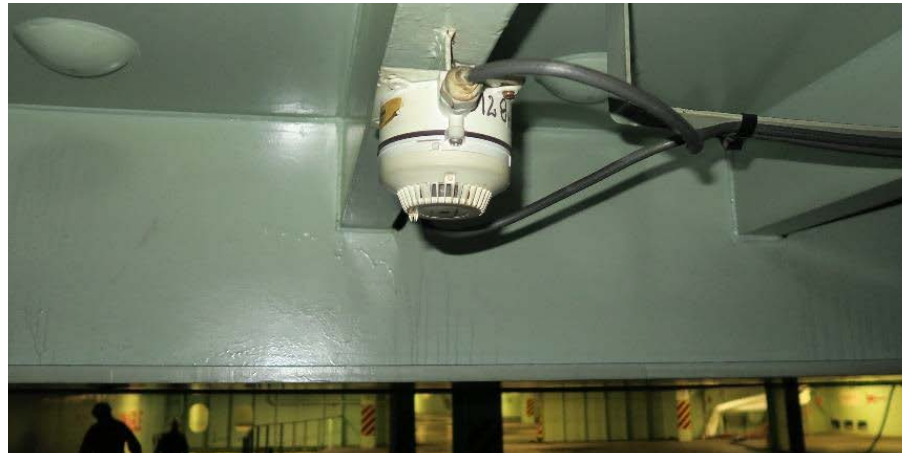
Figure 5. Smoke detector in the cargo hold.
