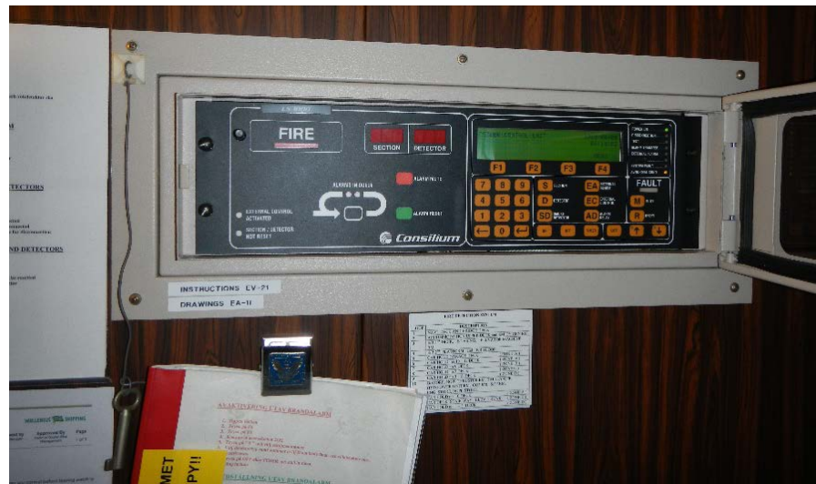
Figure 6. Fire alarm panel indicating which detectors and sections are giving off an alarm. Such panels could be found on the bridge and in the reception.
