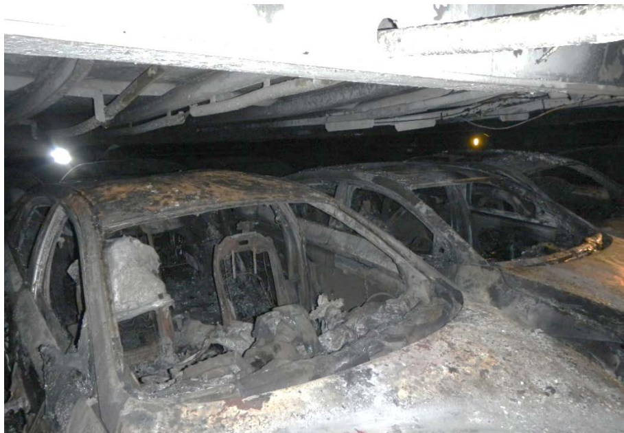
Figure 13. Fire-damaged car on deck 1. Note how the deckhead is bulging downwards.
