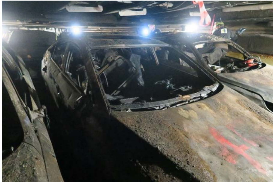
Figure 29. The car with the sunroof, where the fire inside the car affected the hydraulic lines and cables in the deckhead above.
