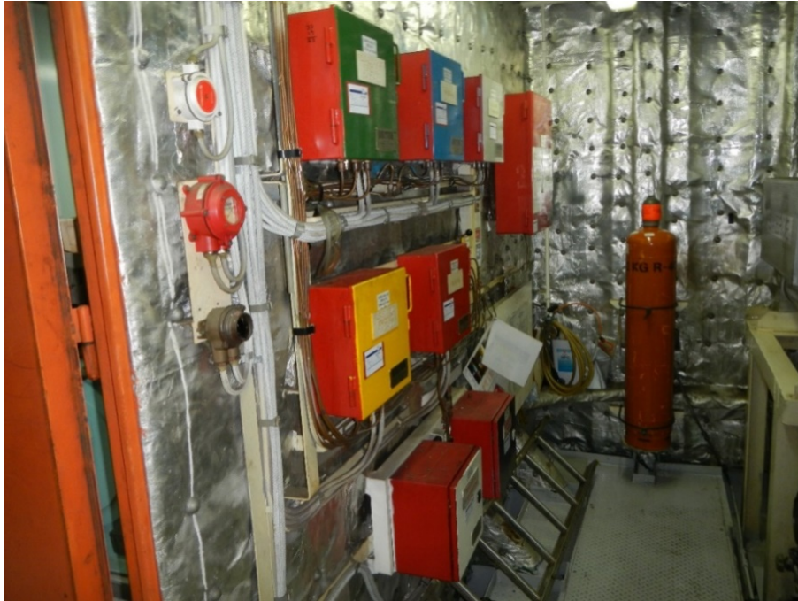
Figure 7. The “CO 2 room” control unit, which was used to set off the fire suppression system.
