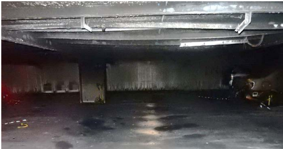
Figure 3. The underside of deck 2, above where the burning cars were standing. The plates and the beams of the deck have been deformed both upwards and downwards.
