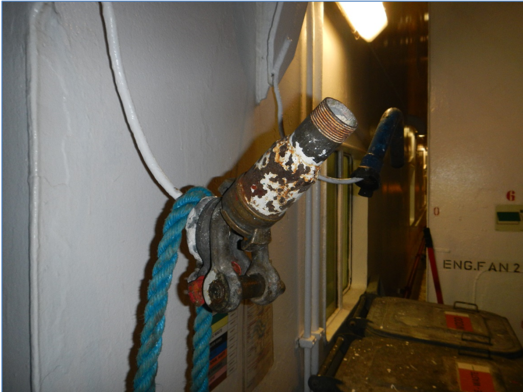
Figure 19. Placement of the water adapter on the bulkhead on the starboard side.
