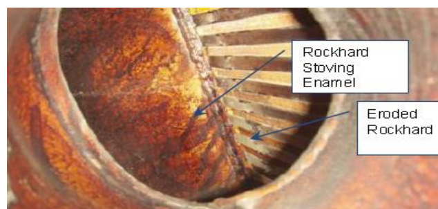
Figure 3. Condenser/Reheater Internal View
