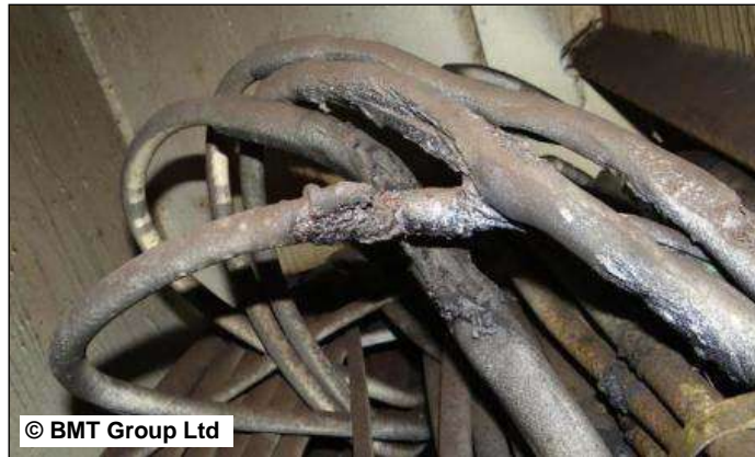
Figure 66: Example of charred cable insulation (1) 39
