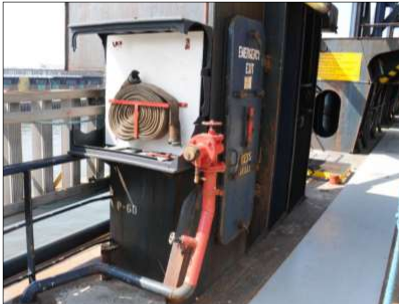
Figure 3: Emergency exit for ro-ro decks 3, 2 and 1 on the main deck
