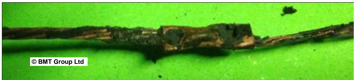
Figure 65: Cable splice with inconsistencies in respect of diameter and number of conductors 38
