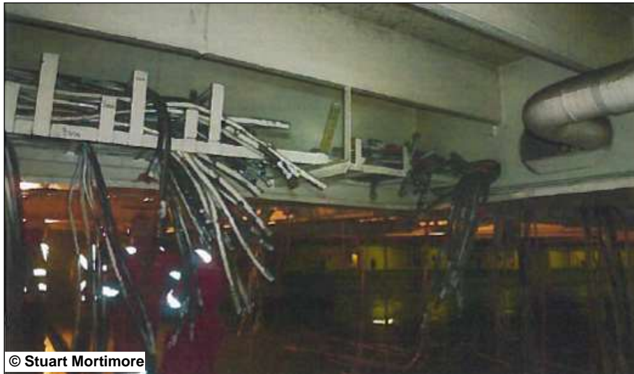
Figure 81: Rear cable splice 54
