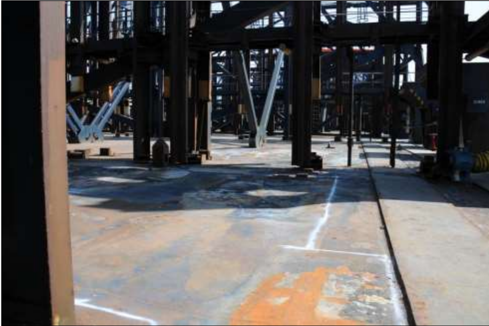
Figure 57: Damage threshold (cargo hold/void space)
