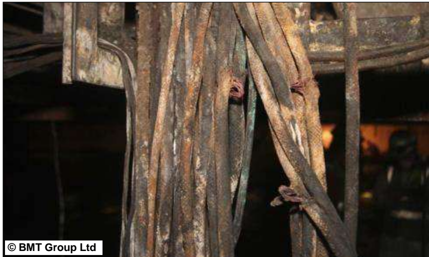
Figure 69: Example of metal conductor protruding from the insulation 42
