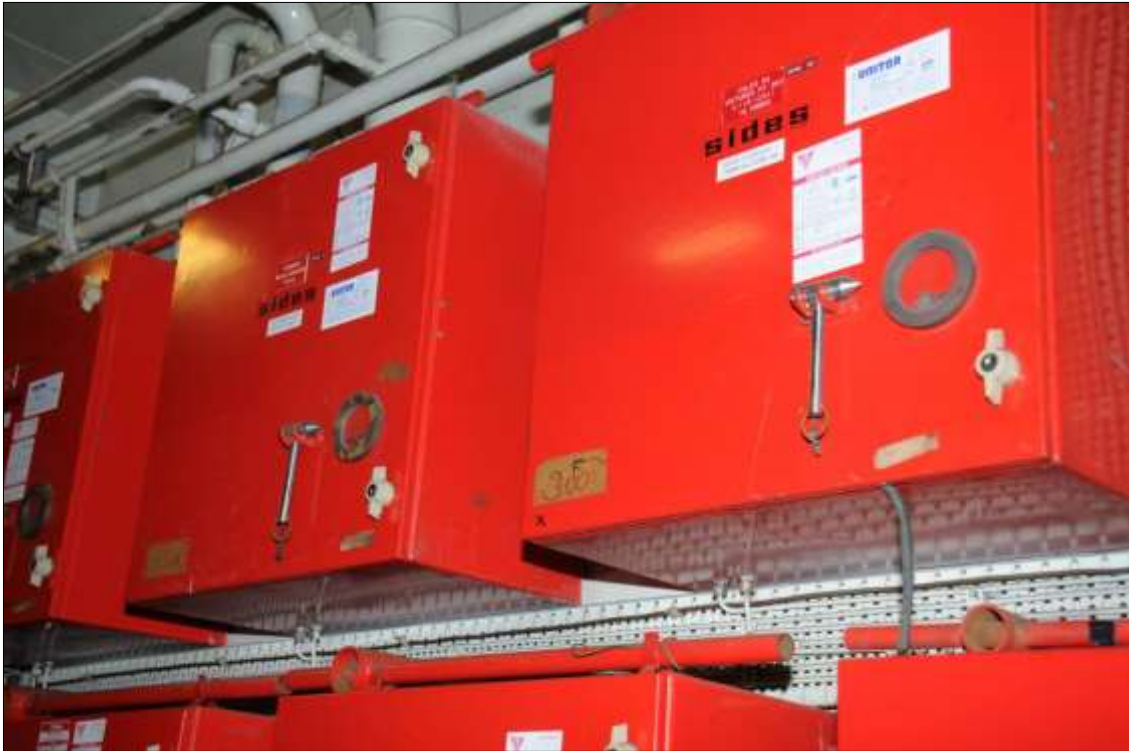
Figure 22: Control boxes for zone 6 (left) and zone 3 A (right)
