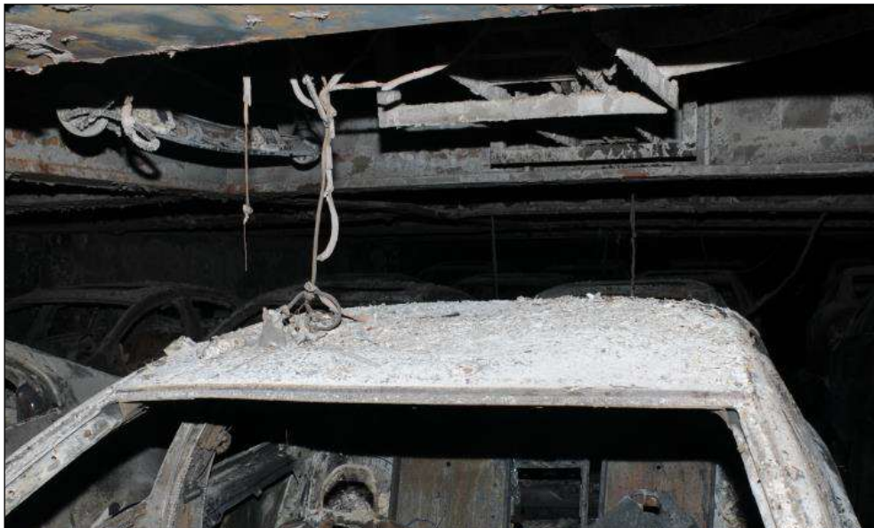
Figure 110: Incompletely burnt cable insulation above car (shielded by the roof of car 4 C)
