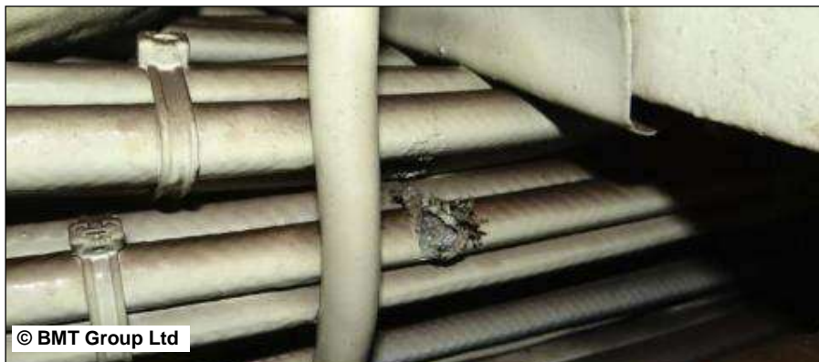
Figure 67: Example of charred cable insulation (2) 40
