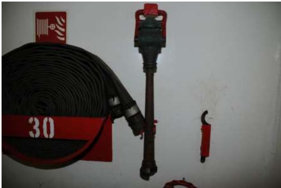
Figure 35: Example of the storage position of a firehose with extinguisher nozzle and coupling spanner on one of the ship's walls
