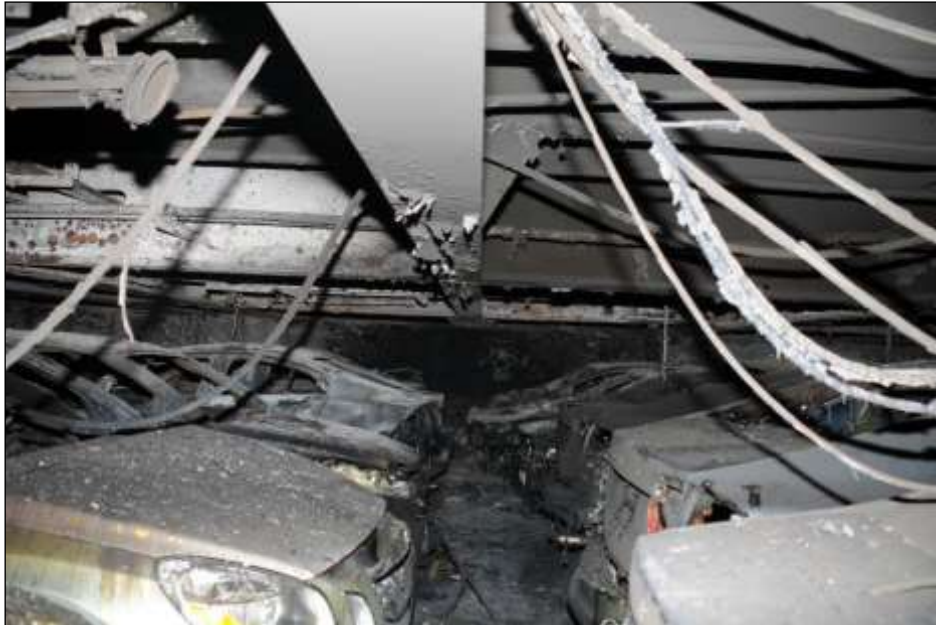
Figure 47: Thermal stress on the deck's ceiling
