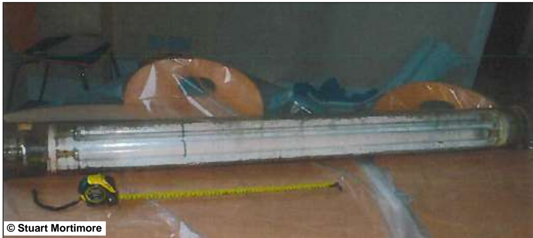
Figure 86: Model of the ceiling light installed in the vicinity of the fire 58
