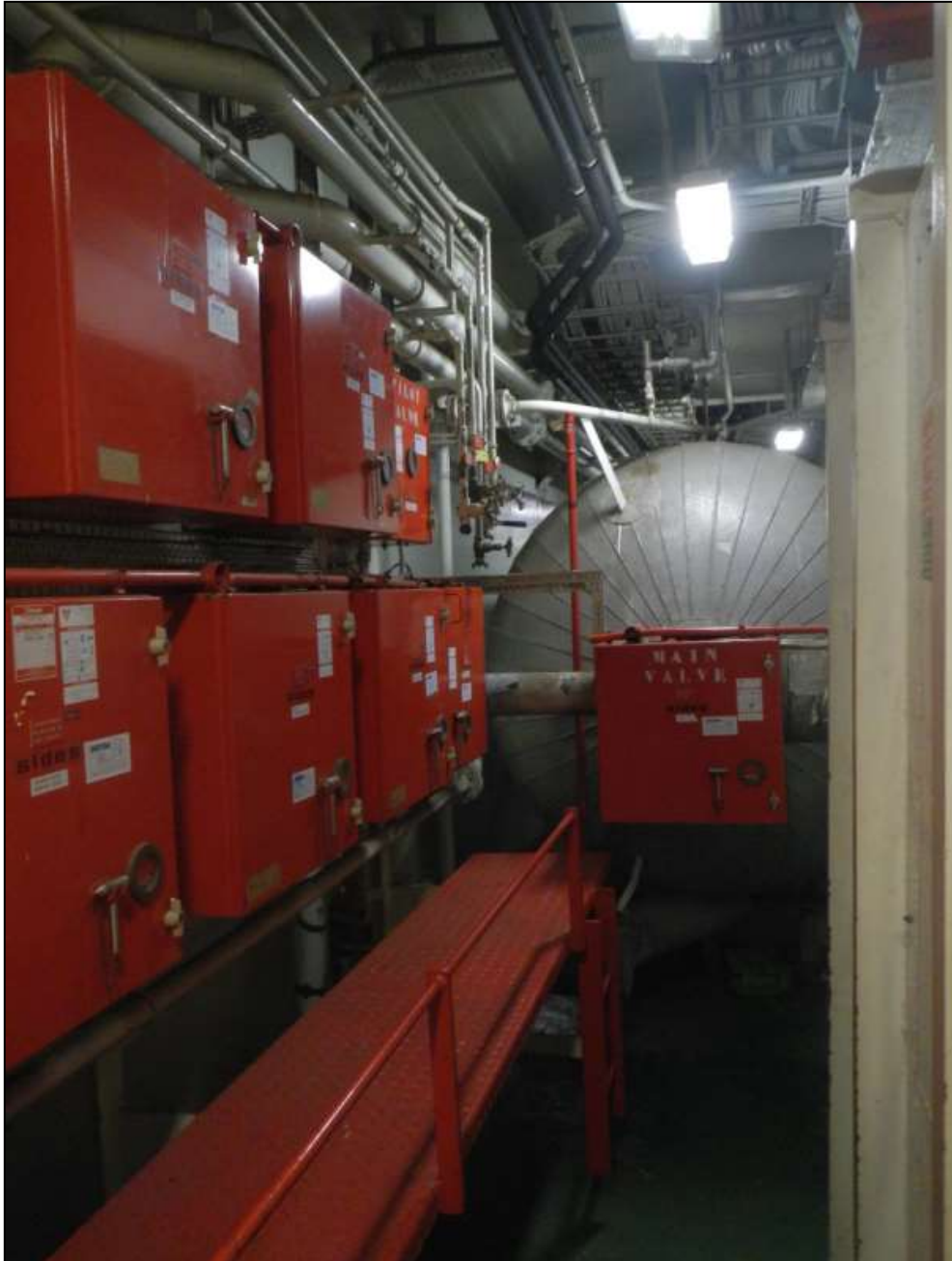
Figure 21: Control boxes for controlling the individual flooding zones (left) 26
