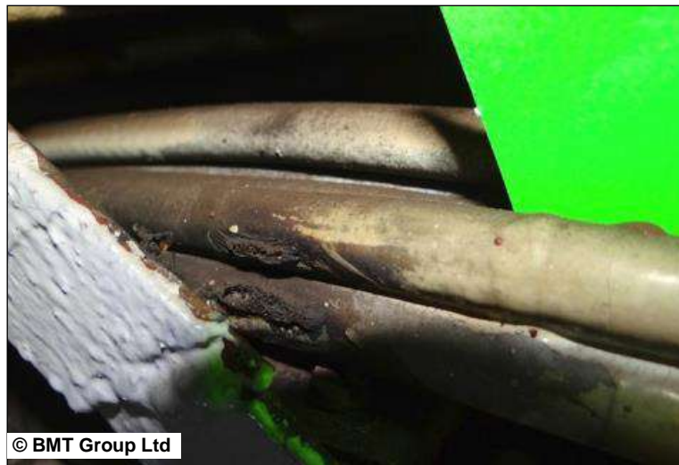
Figure 71: Example of cable insulation damaged by welding operations (1) 44
