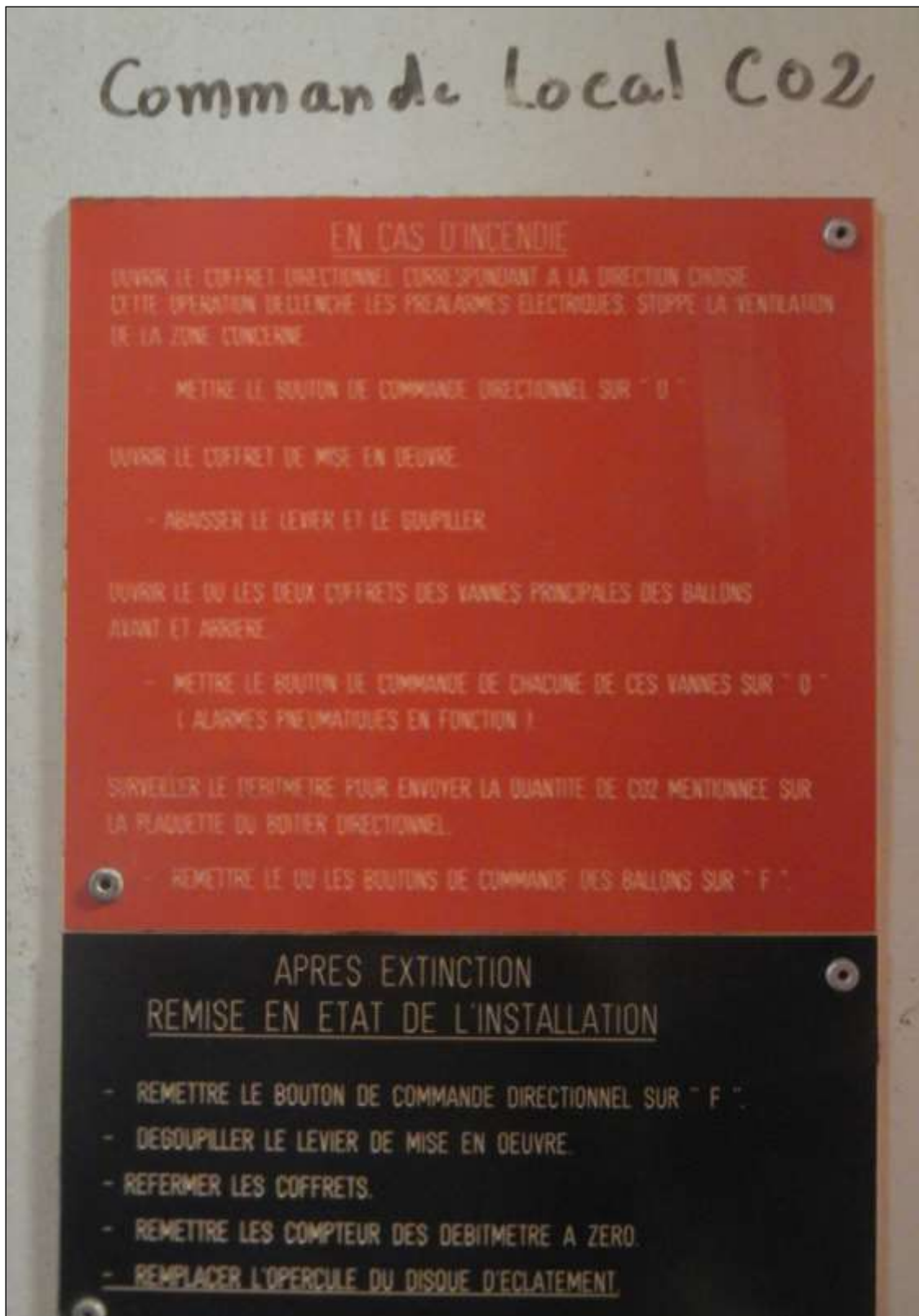
Figure 32: Operating instructions for the local pneumatic release of CO 2 flooding in French
