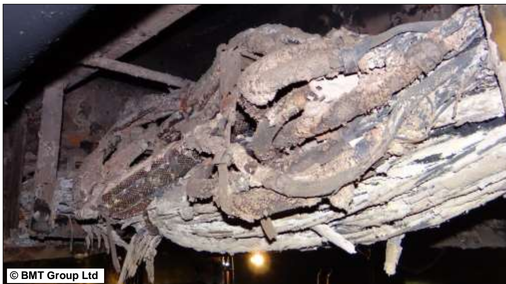
Figure 62: Cable splices on the ceiling of vehicle deck 3 B (close-up) 35
