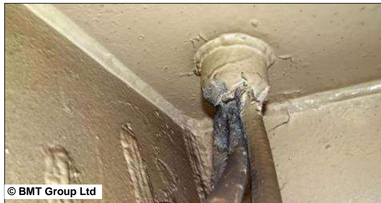
Figure 68: Example of charred cable insulation (3) 41
