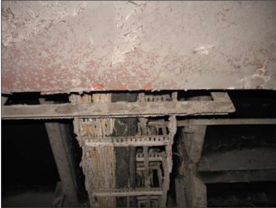
Figure 107: Cable harness above the seat of the fire; uniform fire exposure
