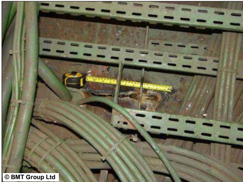
Figure 73: Example of close proximity between welding spot and wiring 46
