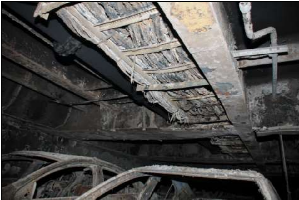
Figure 108: Cable routing above car 4 B
