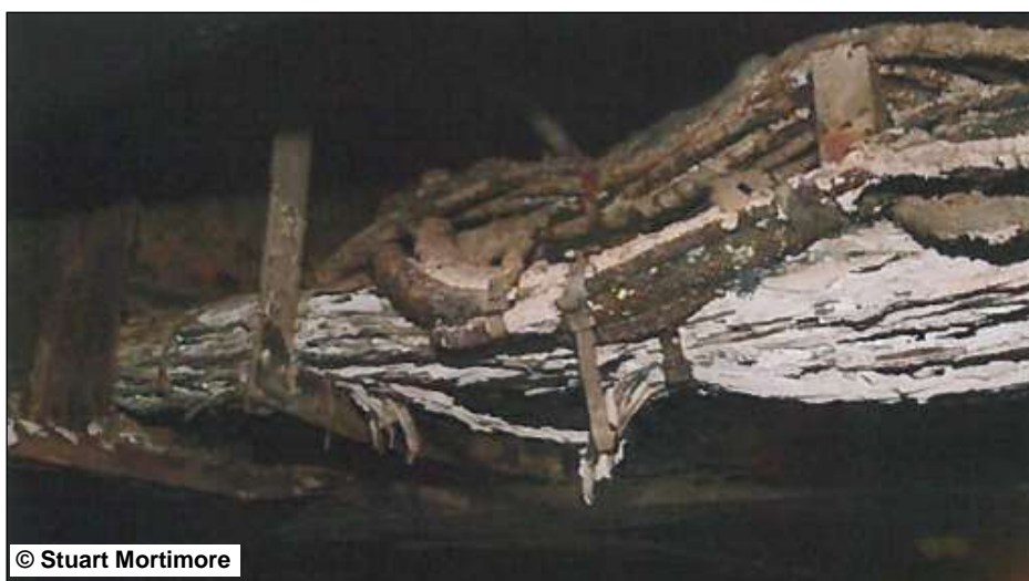
Figure 80: Cable splice above vehicle 5 B 53
