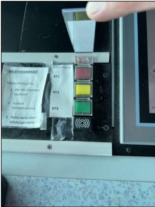
Figure 1. Air traffic controller's alert pushbuttons. (Photo: ANS-Finland)
