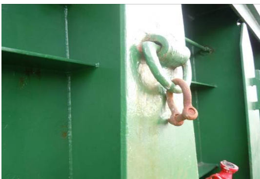
Figure 5. D-ring on hatch frame positioned about 1.1 m beneath the top of the cargo hatch
