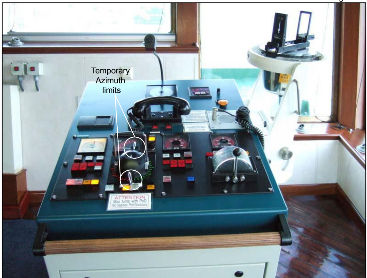
Wheelhouse starboard side console
