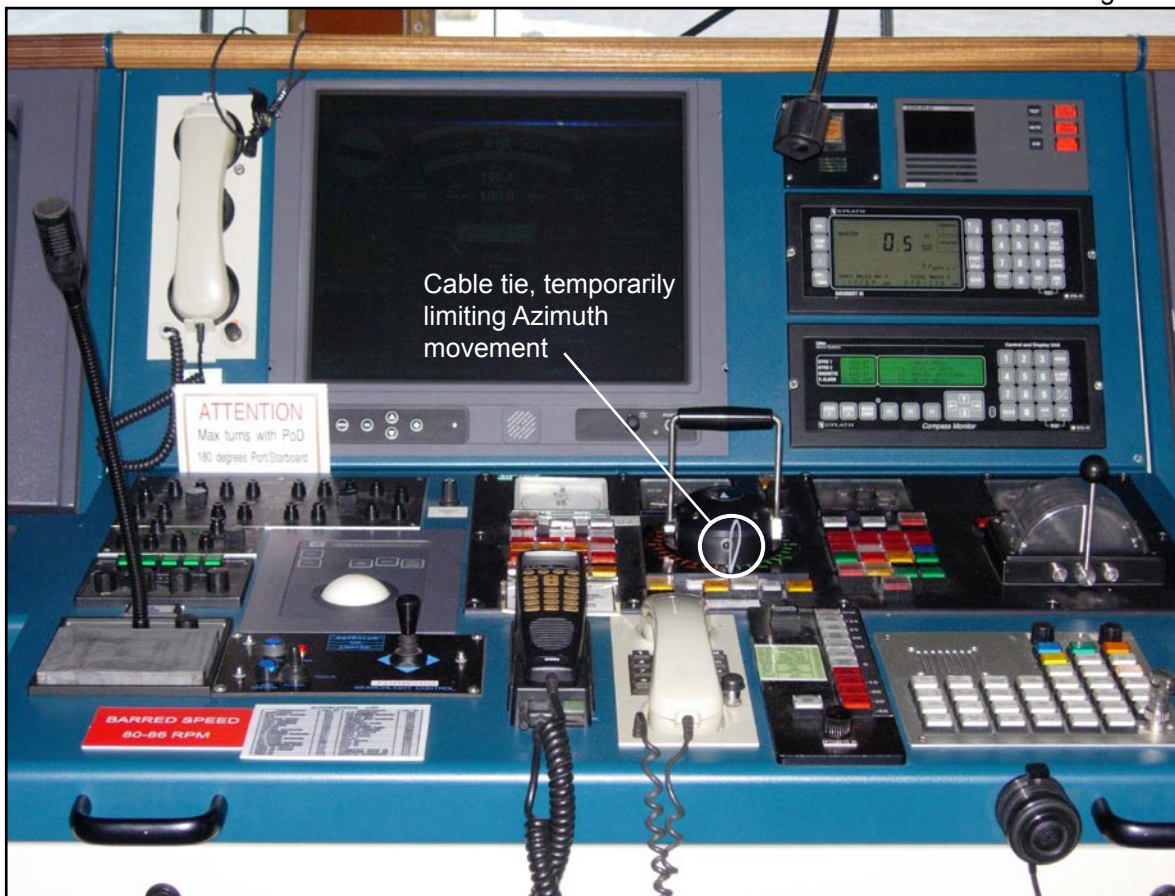
Wheelhouse centreline console
