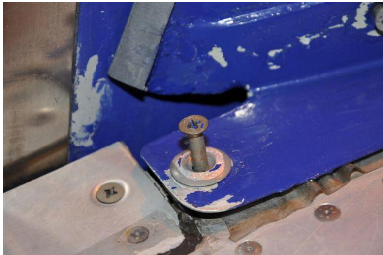
Photo 14: Item 5 (from fig 3) bolt.
