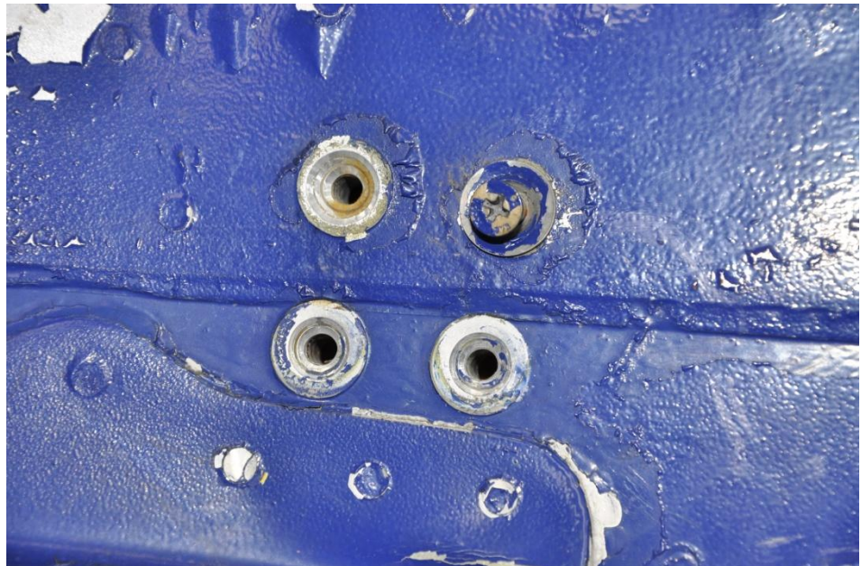
Photo 6: 4-NAS1203-10 location, RH fairing. Showing 1 remaining screw.
