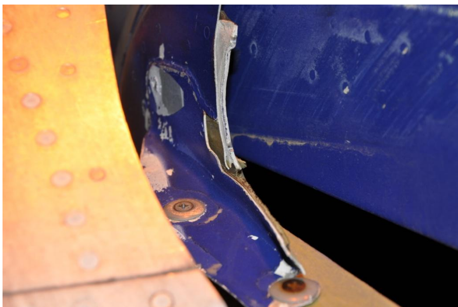
Photo 11: Failed part of fairing still attached to A/C with screws NAS1203-6 and (out of sight) bolt NAS1203-3
