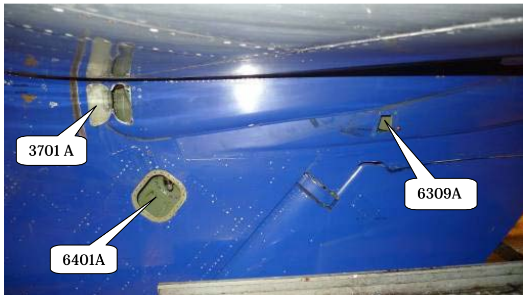
Fig. 6 Opened panels on the left side for lubrication of stabilizer jack screw and stabilizer hinges in accordance with Boeing MD-80 AMM
