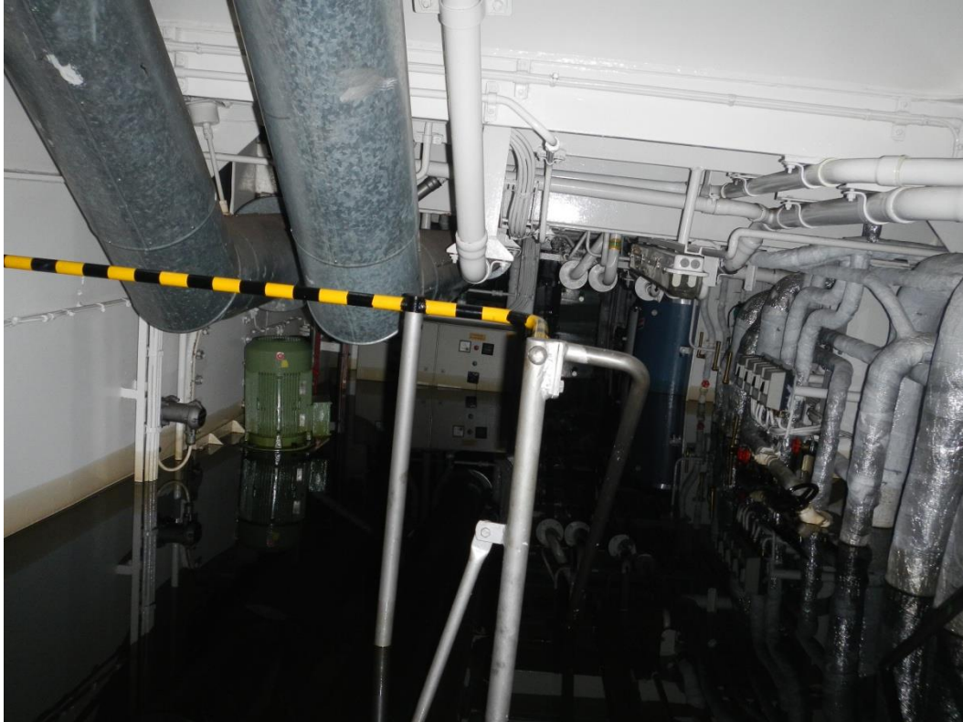
Fig. 2. The engine room after the flooding.
