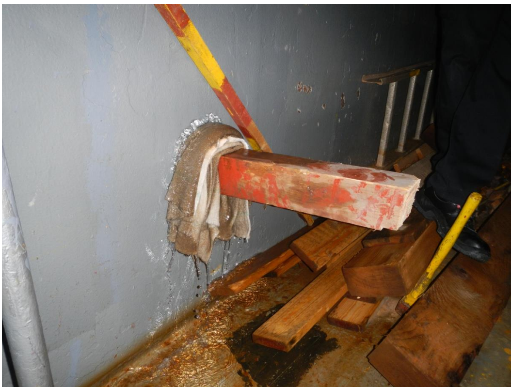
Fig. 6. An attempt to block the flow of water from the engine room. Photo taken from the cargo hold.
