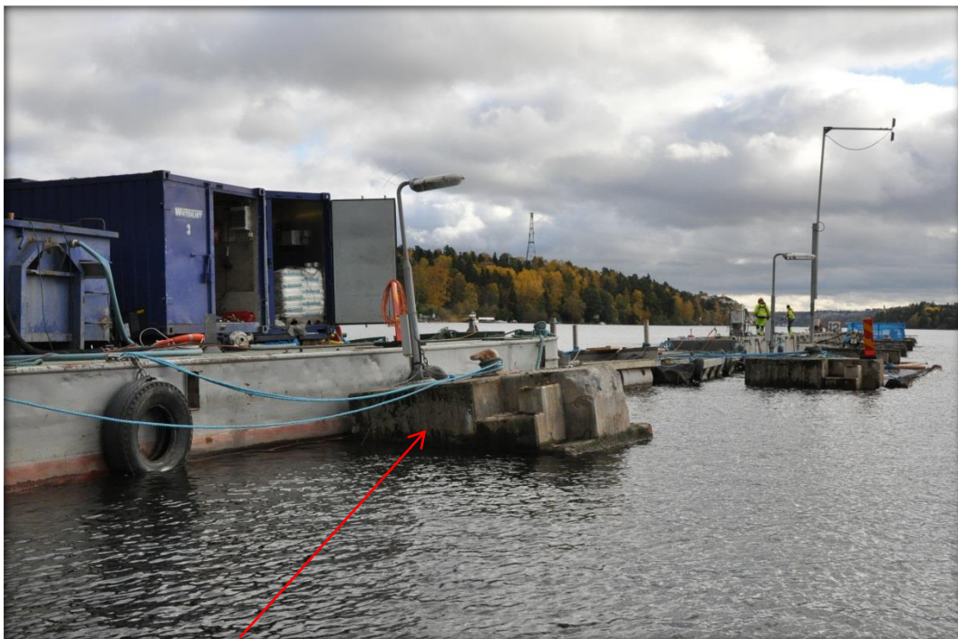
Fig. 4. Fouled dolphin, which was shifted approximately 1.5 m out of position.
