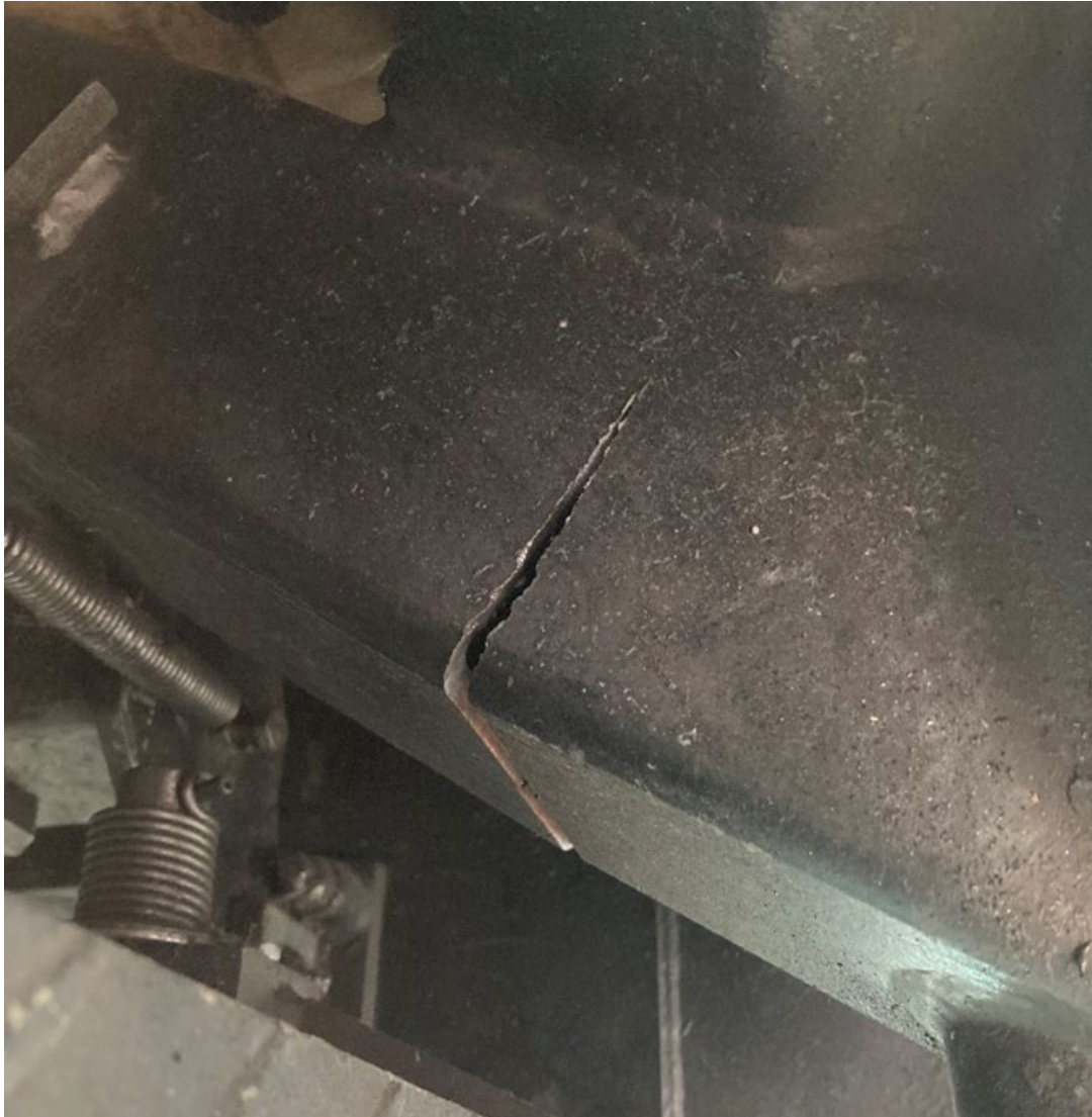
Figure 27. The crack that was discovered on 28 August 2022 in an original rear control arm from 1988. Photo: Gröna Lund AB.
