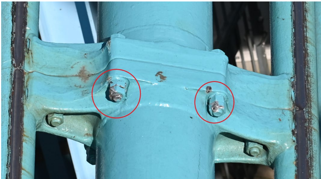
Figure 12. The sites where the impact damage was more severe on the nuts and bolts at the joints are visible within the red circles.
