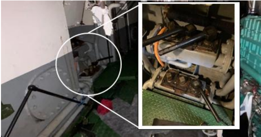
Figure 14. The image shows the bilge box, consisting of two rows with three valves in each. These are connected to several different pipe systems. Image: Klaravik and Swedish Transport Agency (inserted image). Annotations added by SHK.
