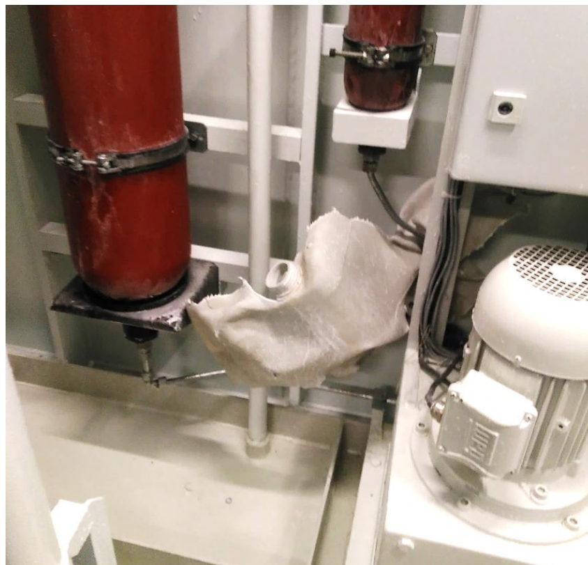
Figure 4: Burst dosing tank as found after the accident 7
