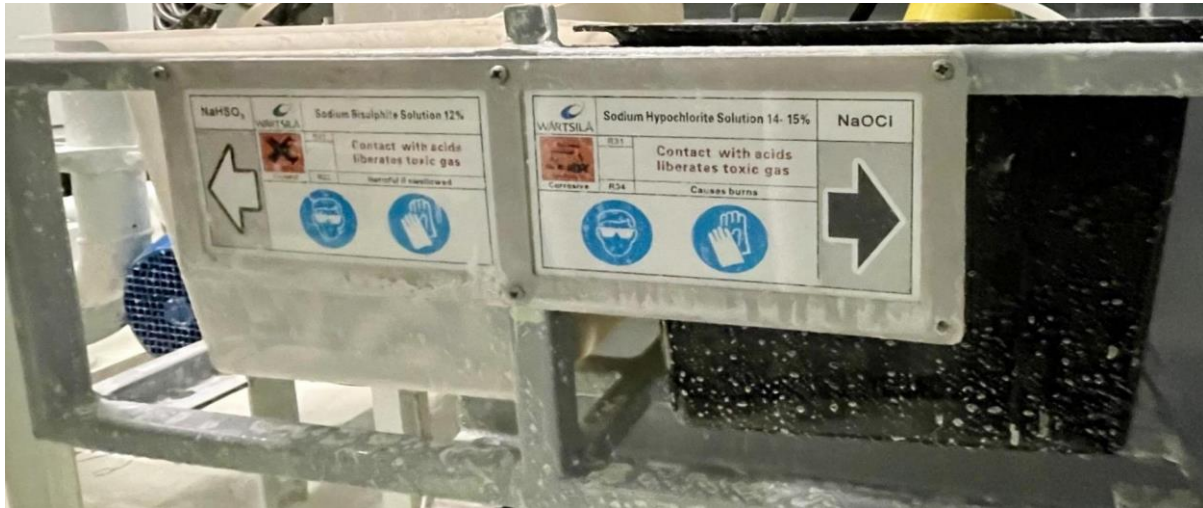
Figure 11: Signs at dosing tanks on CORALIUS 26
