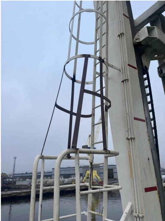
Figure 7. Additional protection has been added between the platform railing and the ladders protective cage. Picture: Wagenborg Shipping B.V.
