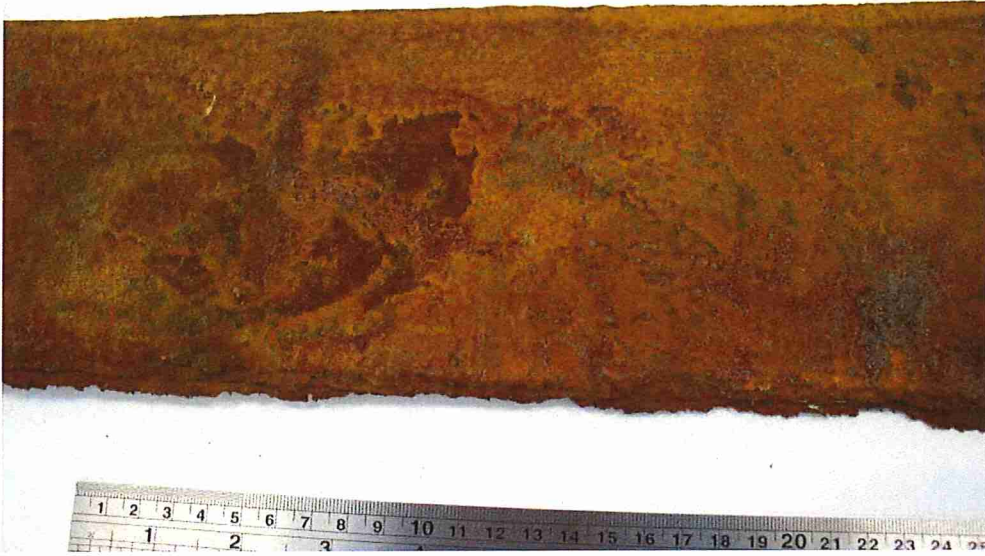
Photo 4. Torn edge of metal strip, view of hull exterior.
