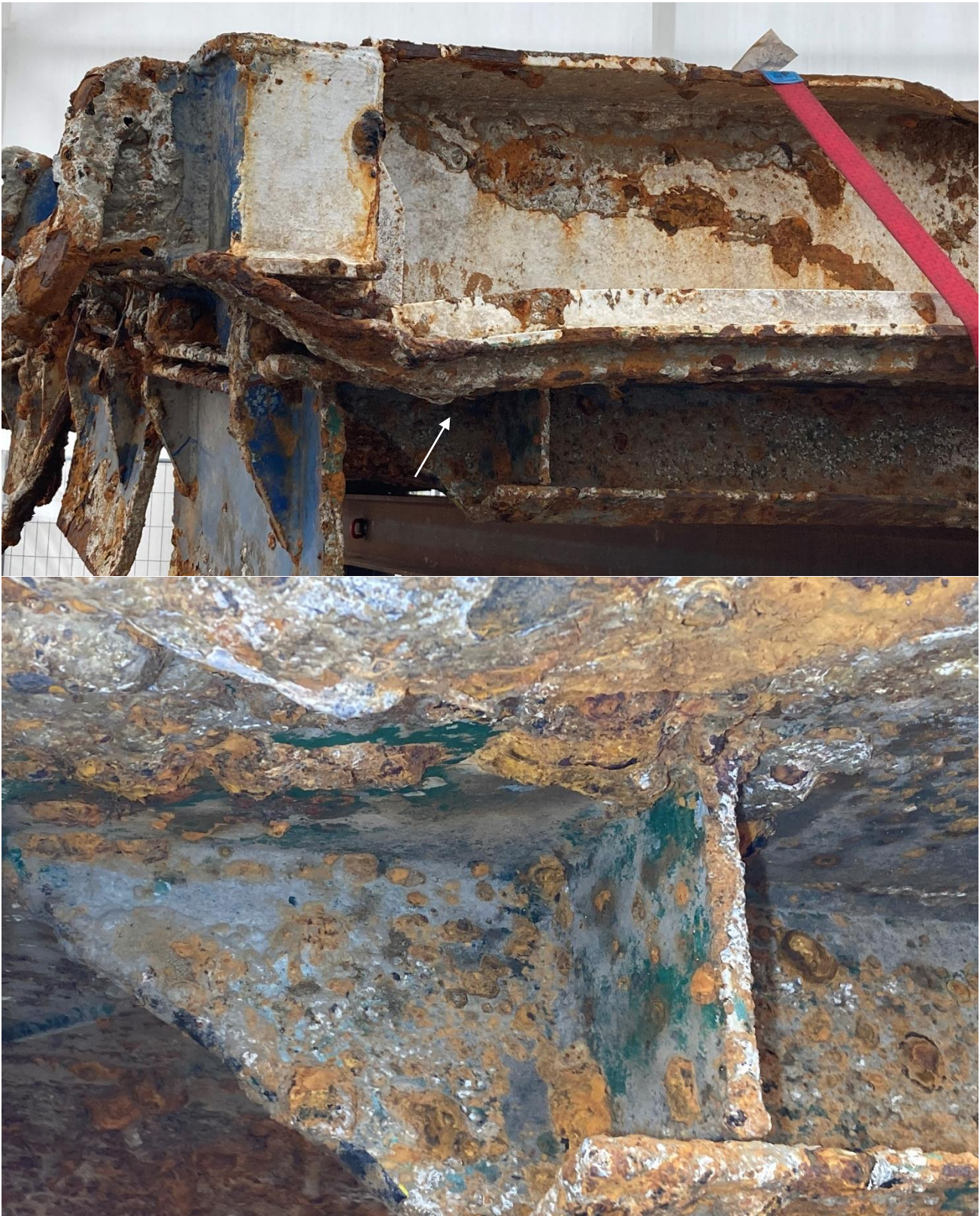
Figure 16. Port side attaching position for railing, no part of the railing remains, the weld has been somewhere below the heavily corroded area (4 in Figure 12).
