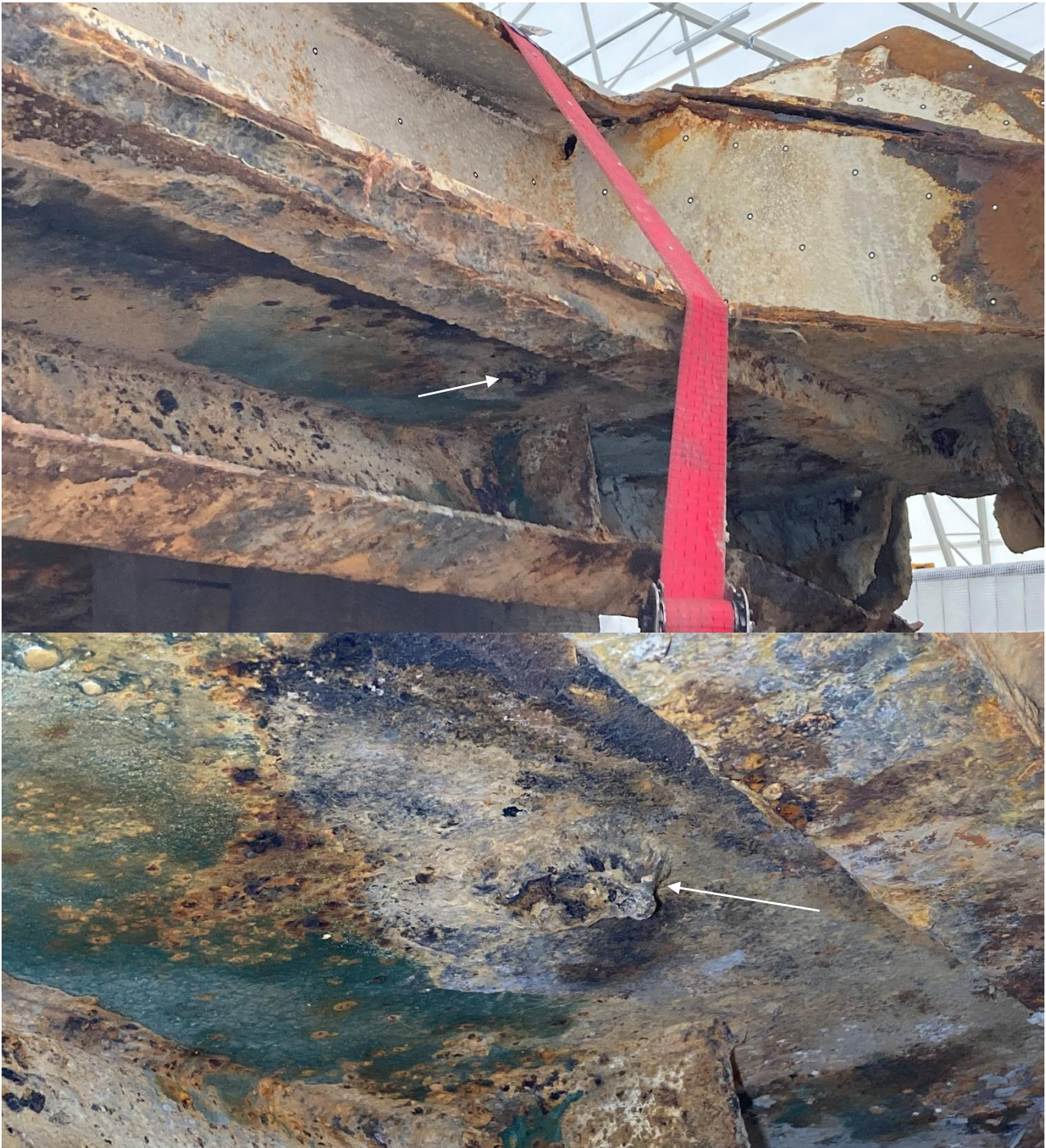
Figure 11. Starboard attaching position for railing, only the weld fillet remains on the bow ramp (3 in Figure 8).
