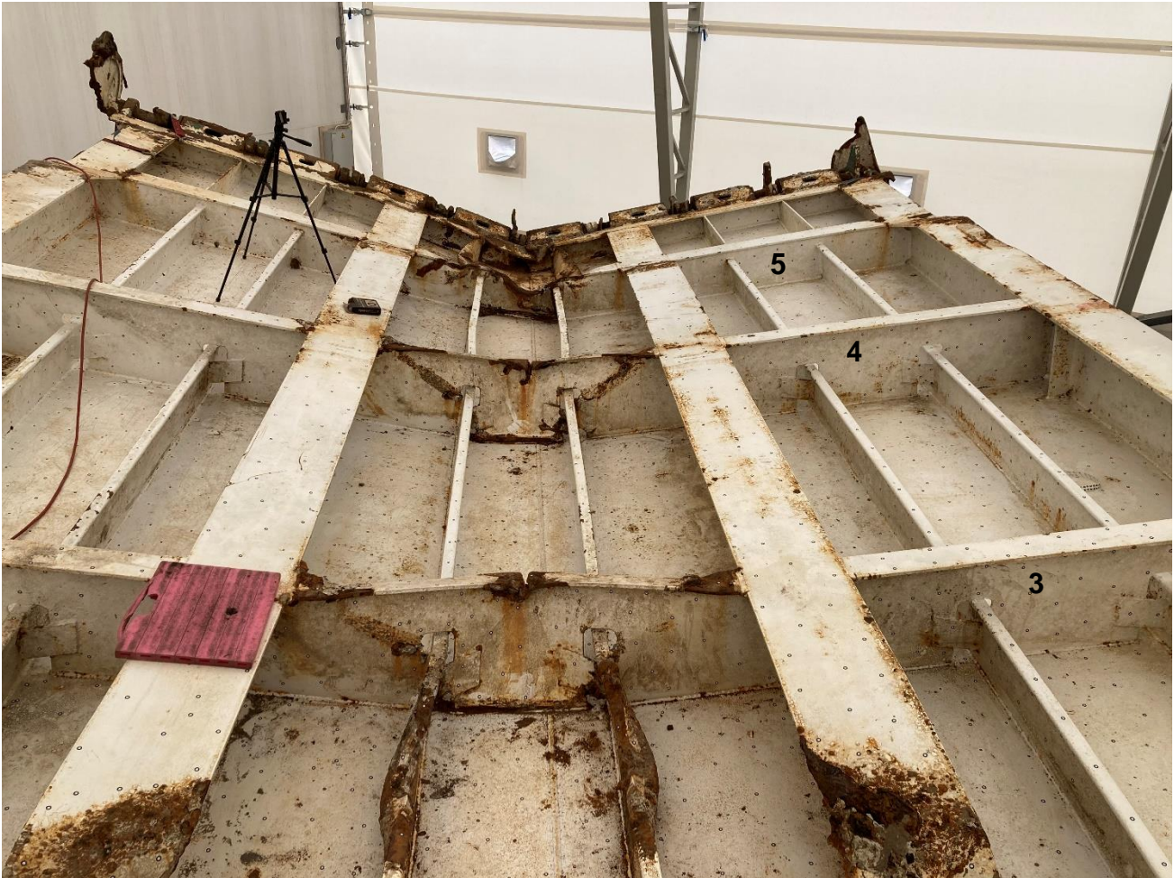
Figure 7. The sea side of the bow ramp seen from the hinge side, transverse beams 3, 4 and 5 marked.
