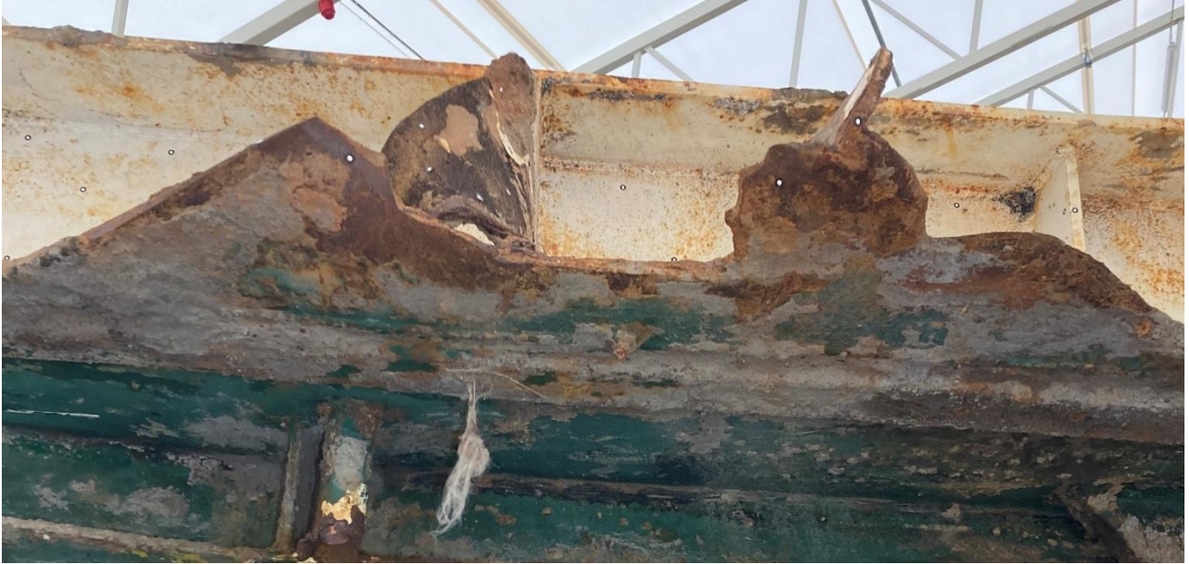
Figure 1. Missing bracket for the ramp locking hook on starboard side.
