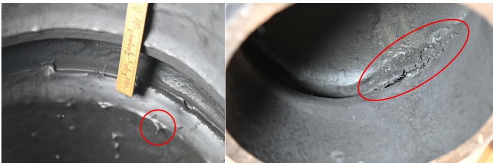
Figure 20. The picture on the left shows the upper side of the joint in the section of pipe where there were drop formations. The red marking shows the drop shape after melted plastic has run down. The picture on the right shows the opposite side from the drop formations in the joint. The carbonised remains where the plastic has probably burned is visible in the red marking.
