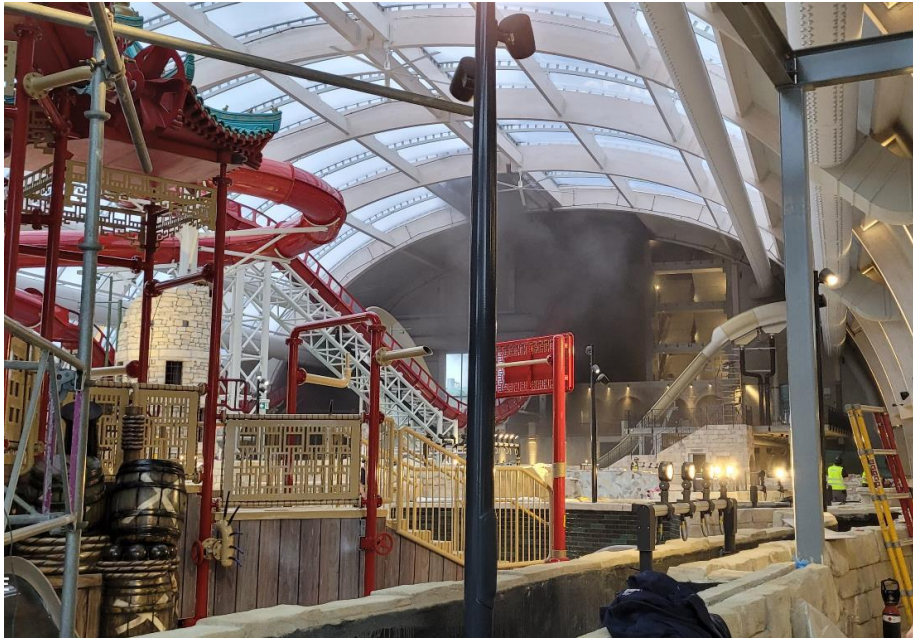
Figure 6. At 10:06 hrs the tower was filled with smoke and smoke began spreading to the pool building. Photo: EnviroProcess Sweden AB.
