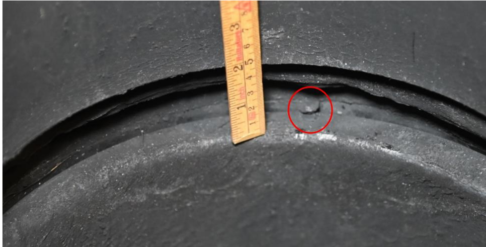
Figure 19. The joint on the inside of the electrofusion coupler with a gap of c. 45 mm between the pipes. The red marking indicates the heel. Melted plastic that is being forced out is visible at the upper edge of the joint.
