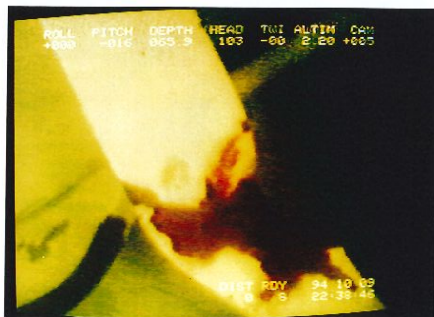
Figure 8.12 Indentations on a beam on the lower side of the ramp.
