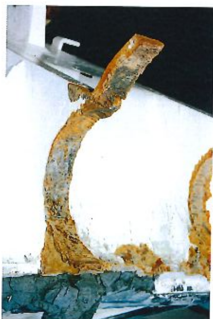
Figure 8.23 Failed port lug of visor starboard hinge.
