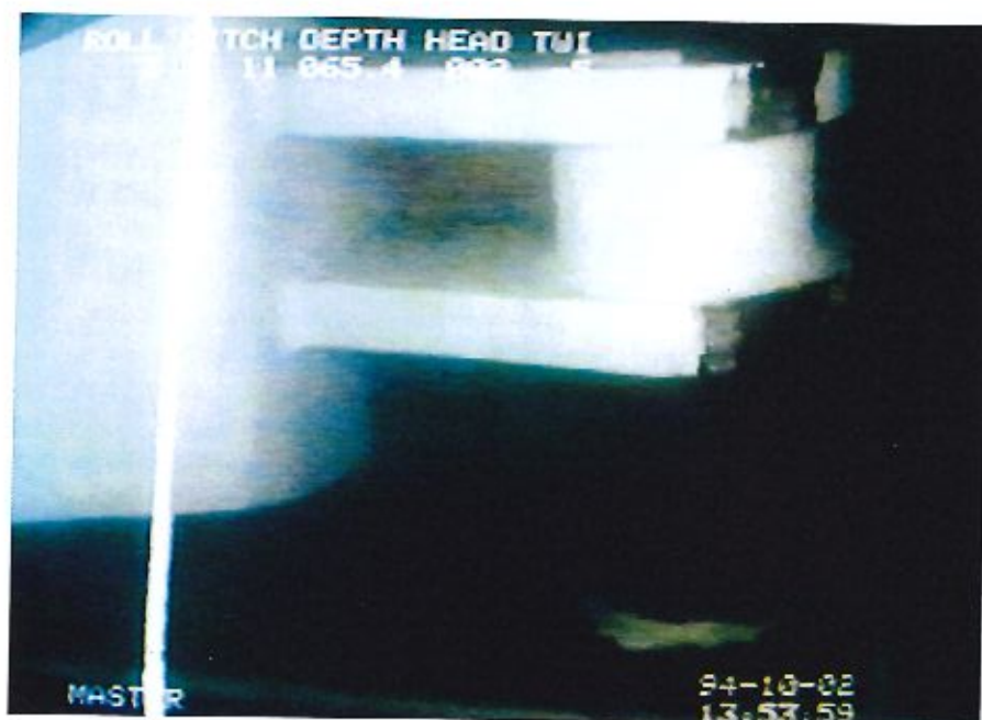
Figure 8.16 Deck hinge fitting, port side. One separated hinge bushing visible at bottom picture.
